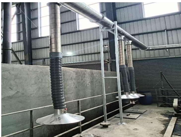
沥青乳化罐加热、搅拌废气集气罩
